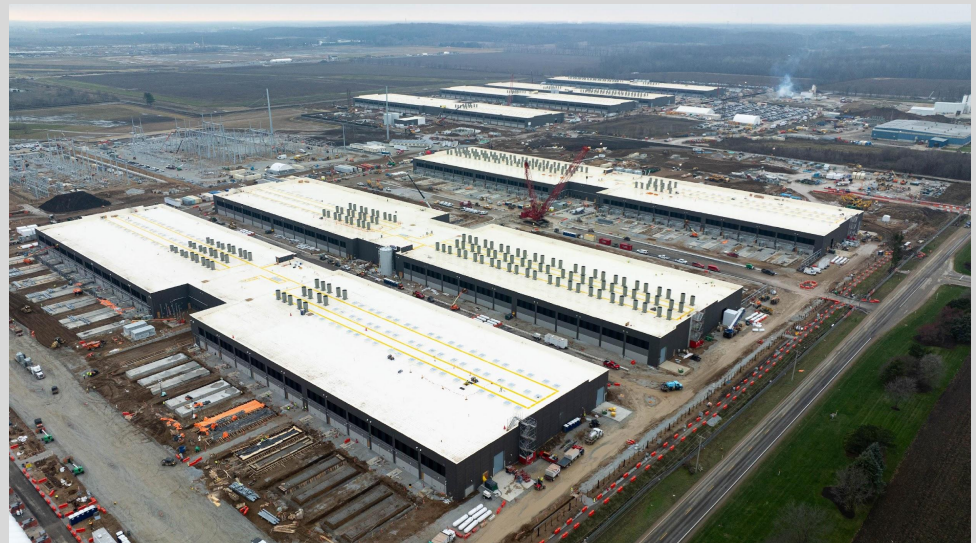
Photo: Amazon data center being constructed in New Carlisle, IN. Credit: Michael Clubb / South Bend Tribune
