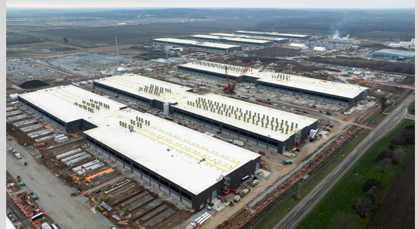
Photo: Amazon data center being constructed in New Carlisle, IN. Credit: Michael Clubb / South Bend Tribune
