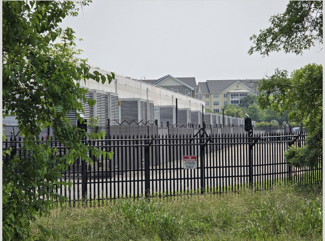
Photo: Backup diesel generators at a data center (foreground) adjacent to a retirement community (background). Credit: Ben Inskeep | CAC
