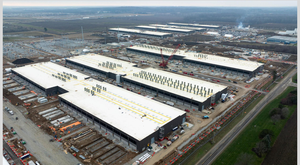
Amazon data center being constructed in New Carlisle, IN. Photo: Michael Clubb / South Bend Tribune
